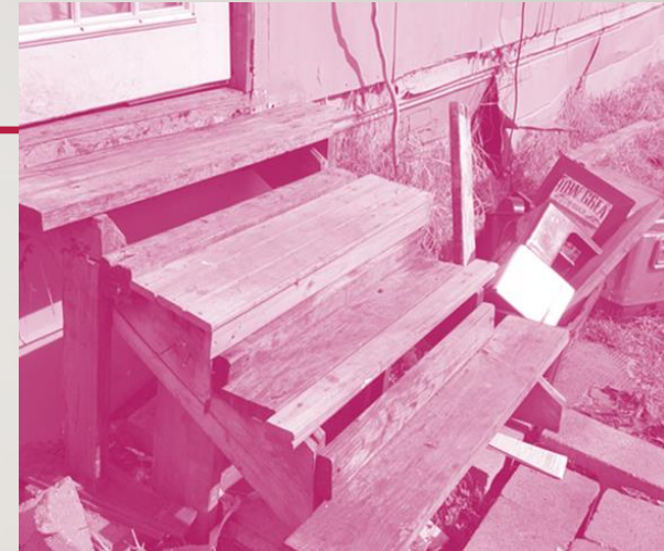
EGRESS & INGRESS HAZARDS
